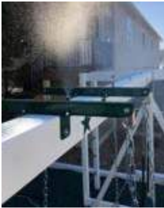
Swing Beam Misting System
